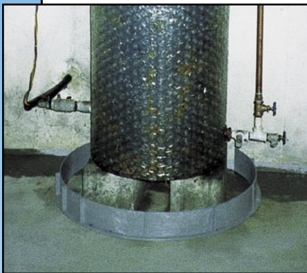
FloodRing™ around a water heater protects your basement from leaks and flooding.
